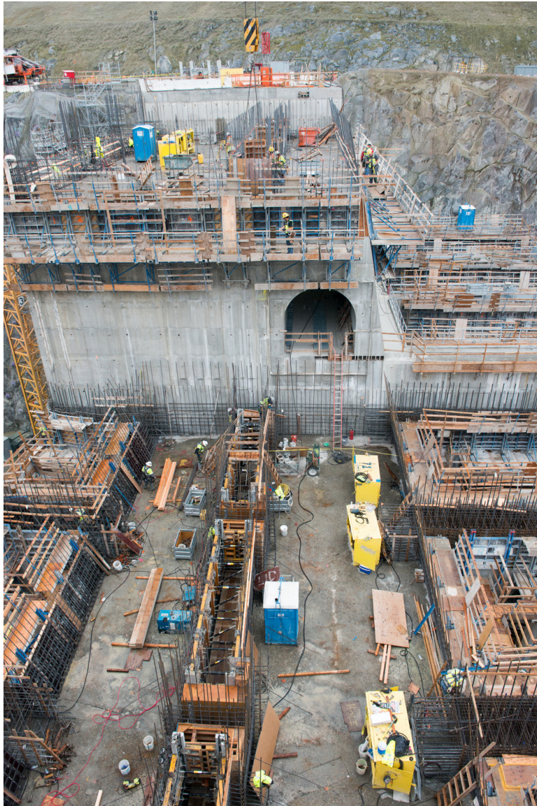
The Folsom Dam auxiliary spillway construction site on February 26, 2014. Photo Credit: Courtesy of California Department of Water Resources, Florence Low
