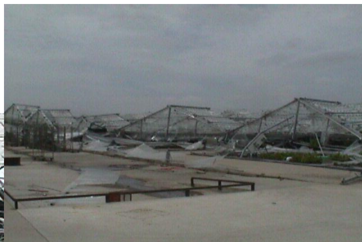
Greenhouses destroyed by tornado about 2 miles southwest of St. Elmo, Illinois.
