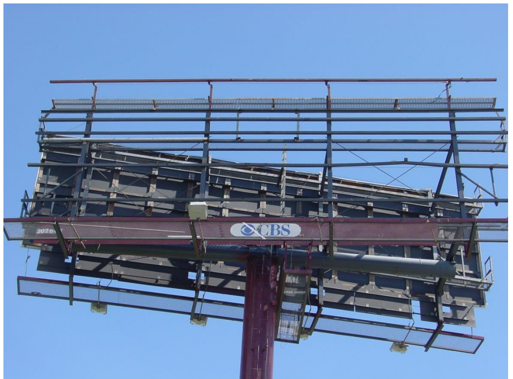
Sheet metal blown away from the supports of a large sign off of Interstate 64 and just west of Jefferson Avenue. Viewing up and to the east.
