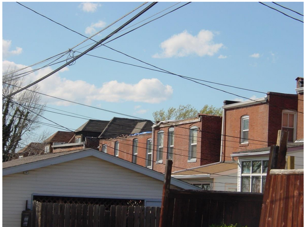
Roof damage to three structure on Blaine Avenue approximately 150 yards west of Grand Ave. Viewing west northwest. Three witnesses observed roofing material rising vertically into the funnel.
