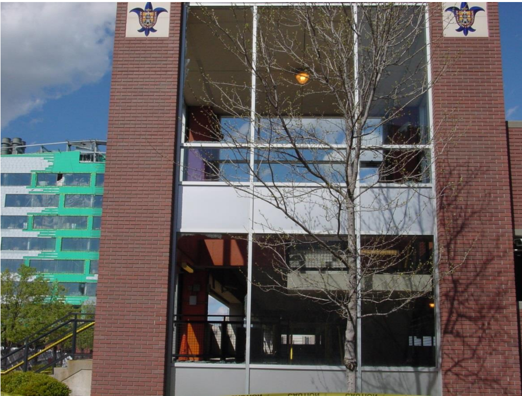
Windows blown out at one of two parking garages on the south campus of Saint Louis University. Viewing north.
