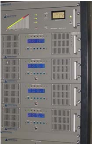
New, solid-state, NOAA All-Hazards Radio transmitter on Stone Mountain, GA.
