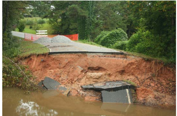
Road washed out by flooding during the epic September 2009 event.
